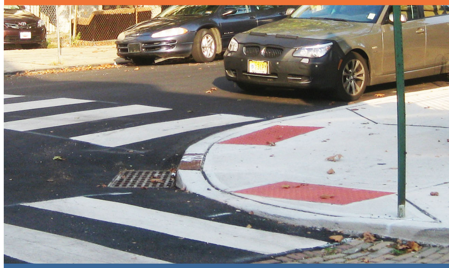
Intersections should have two perpendicular, ADA compliant curb ramps per corner.
