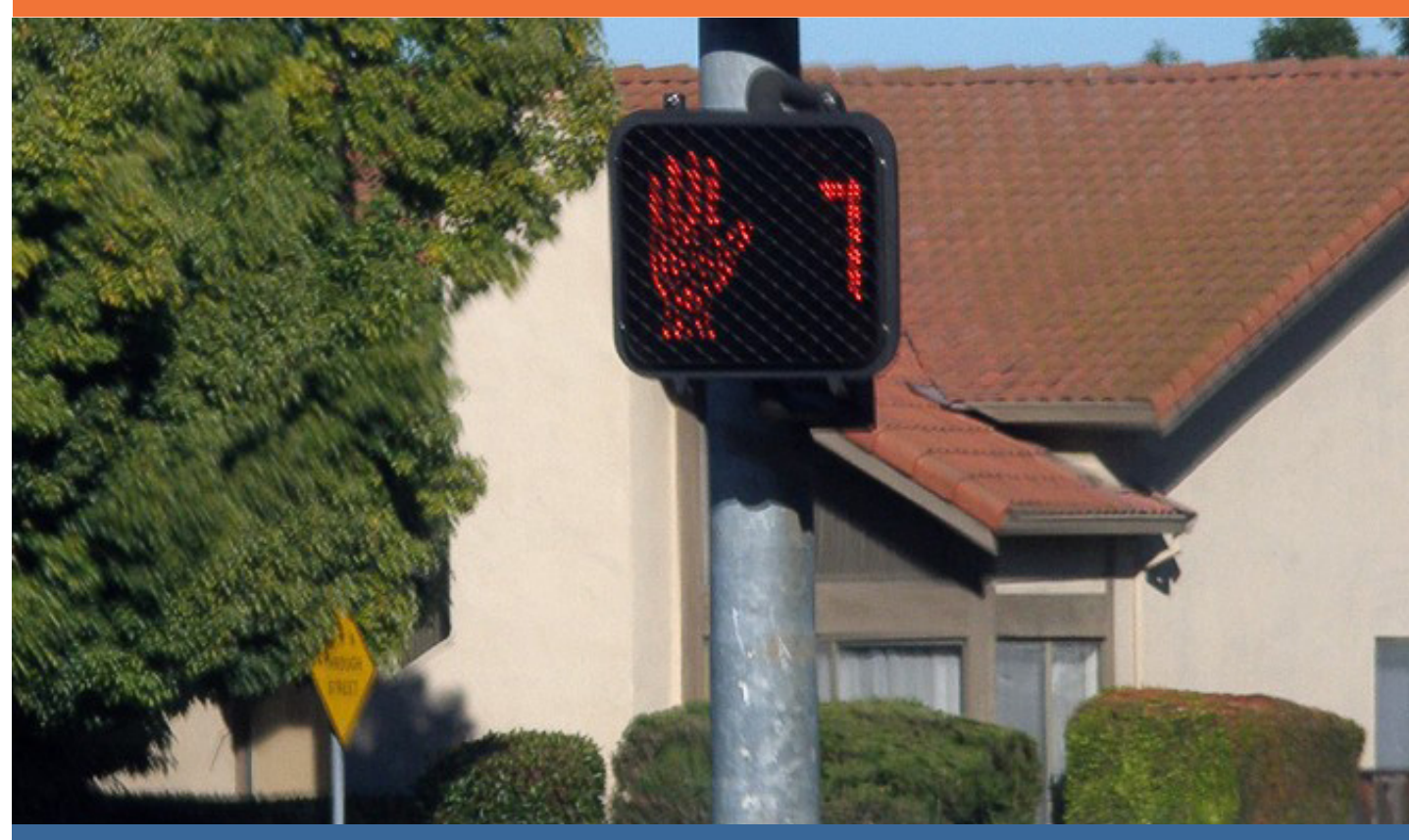
A pedestrian countdown signal displays the number of seconds remaining until the signal changes.
